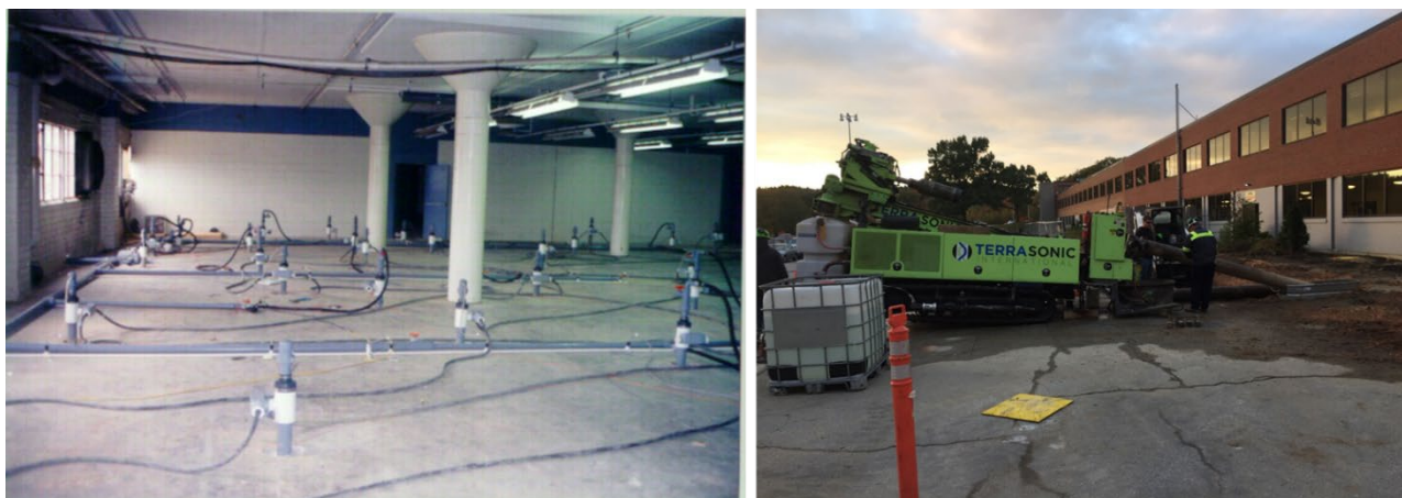
Figure 17. Thermal remediation systems have been installed vertically in warehouses where there is access for a drill rig and under active manufacturing buildings using angled borings.
