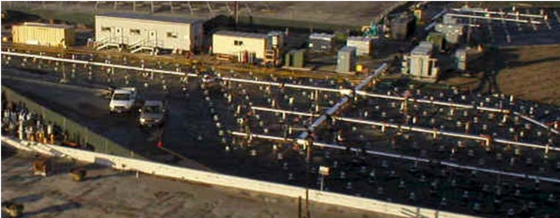
FIGURE 3. ISTD well field and process equipment, Alhambra, CA.
