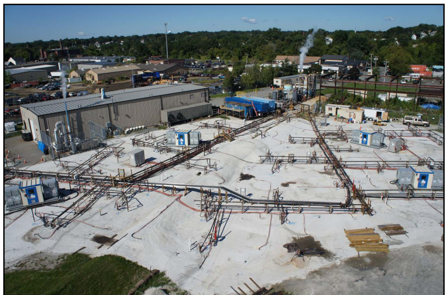
Aerial view of the ET-DSP™ wellfield in operation
