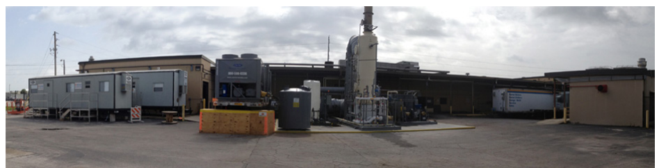
A view of the thermal process equipment
