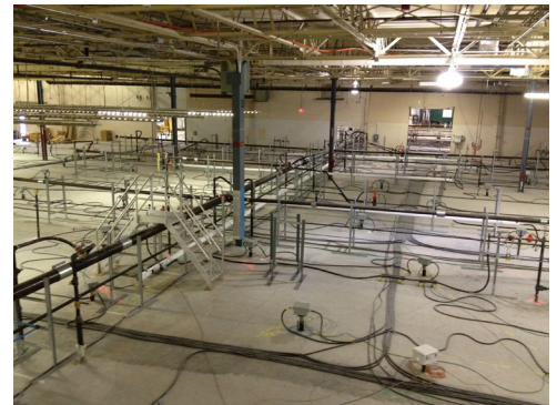
Partial view of ISTD/SEE wellfield inside building
