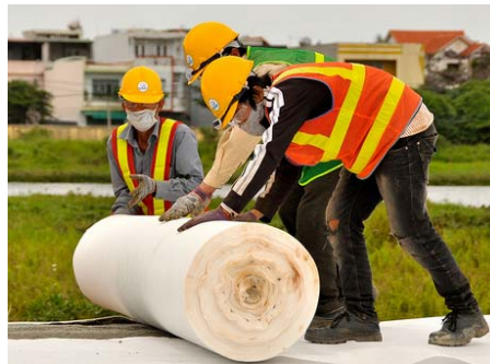
Installing the liner of the drying pad foundation (Photo: R. Nyberg, USAID)
