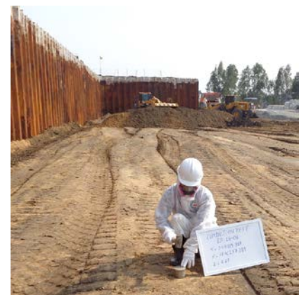
Testing compaction of soil/sediment placed in the thermal treatment structure (Photo: CDM Smith)
