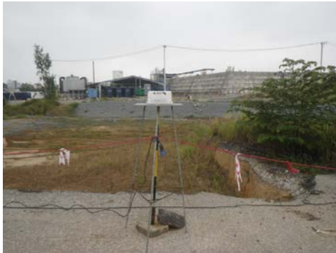
Dust monitoring while moving contaminated soil/sediment from stockpiles to the thermal treatment structure (Photo: CDM Smith)
