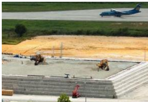
USAID contractors excavate dioxin-contaminated soil and sediment and place it into the containment structure for thermal treatment at Danang Airport. (Photos: USAID and TetraTech)
